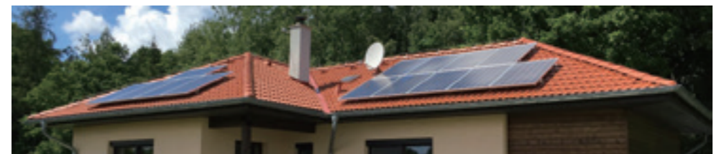
ENERGY STORAGE SYSTEM
